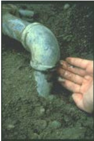
Leaking pipe from UST
