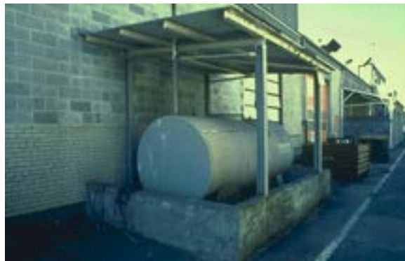
Covered AST with secondary containment
